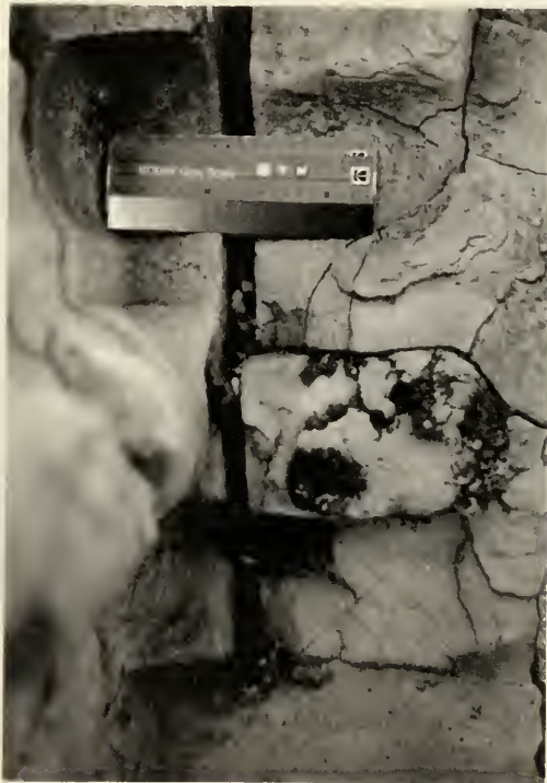
Fig. 21. Biological growth on tuff at intersection of west wall of nave and transept adjacent to open joints and cracks (Photo: Anne Brackin).
